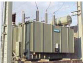
EnBW AG , Siemens Dresden, Germany
