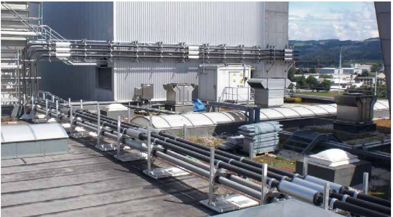
Our busbars in use at the power plant Gud Linz
